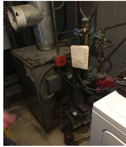
The previously installed, Utica BC Oil Fired Hot Water Boiler in the laundry room of the Rosati home, which operated for over 50 years.
